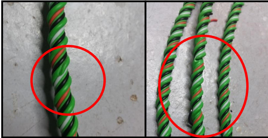
Figure 15: Cable break alarm due to broken wires
