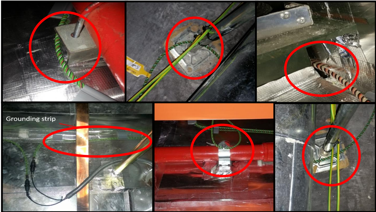
Figure 13: Leak false alarm due to the contact with metallic parts
