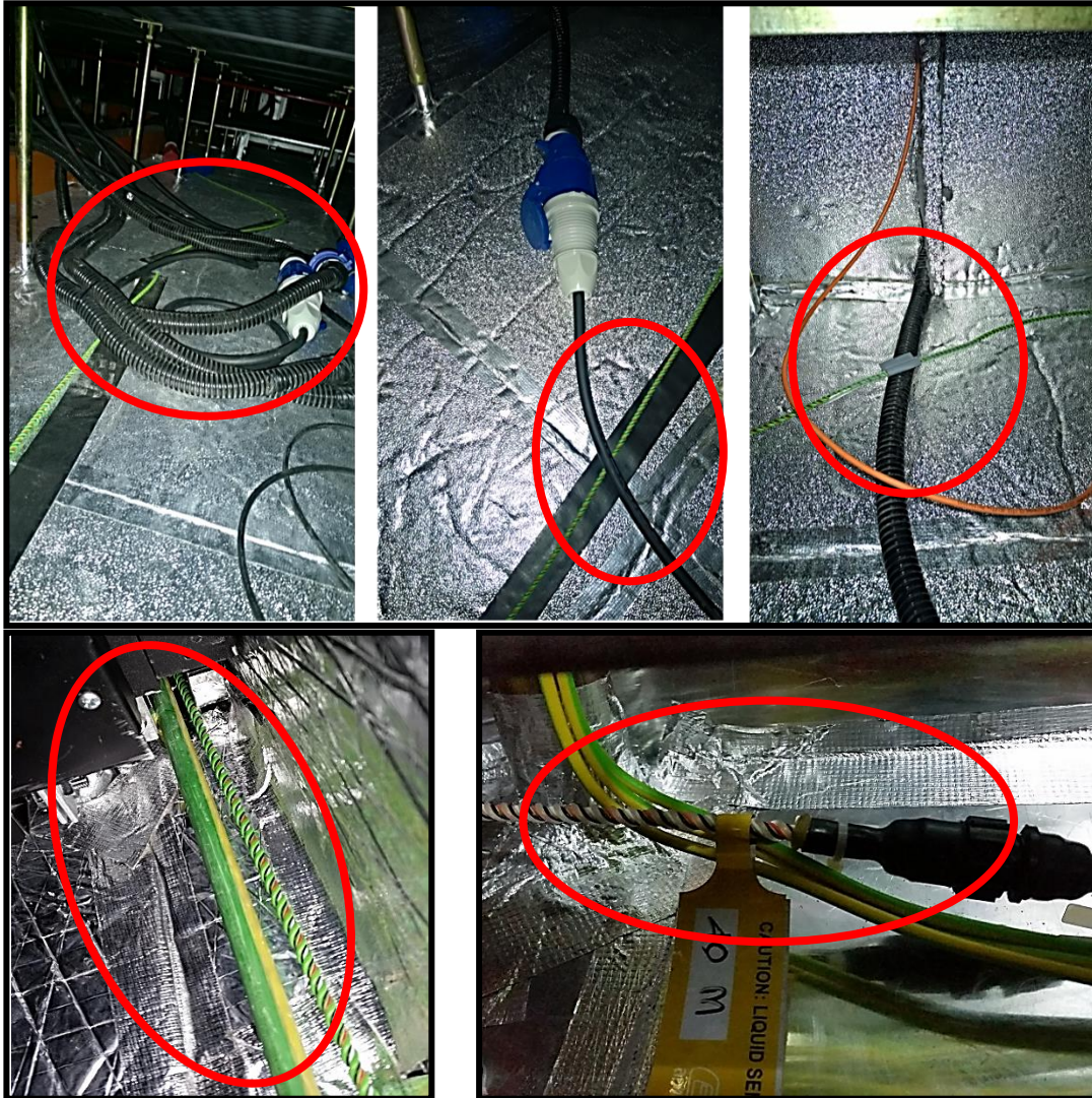
Figure 19: Leak false alarm due to EMI from nearby High Voltage cables
