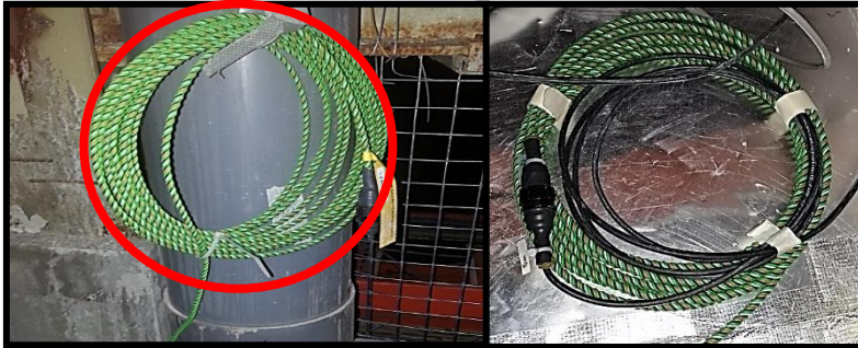
Figure 17: Leak false alarm due to coiling of excess sensing cable
