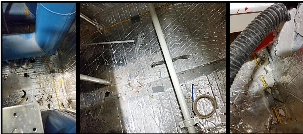
Figure 20: Leak false alarm due to general dirty site condition
