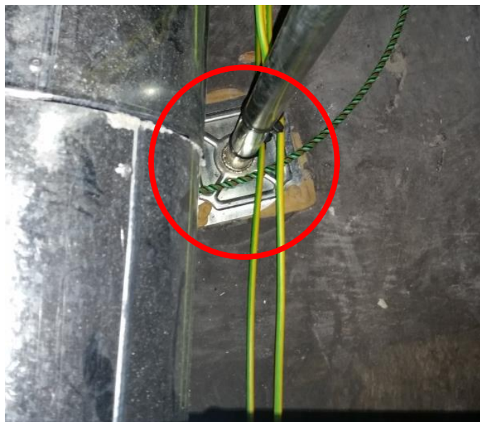
Figure 16: Leak false alarm due to sensing cable touching metallic parts
